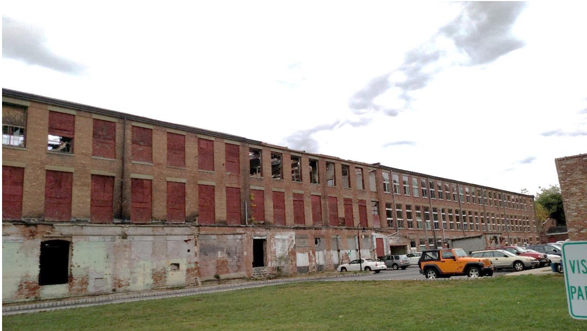
Photo 5: View to the north of Building 16 which is located adjacent to Building 10. Building 10 is currently residential apartments.
