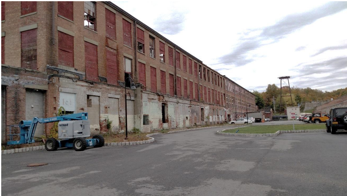
Photo 4: View to the north of Building 16. The existing structure is unsound, and will be replaced with a similar style building.
