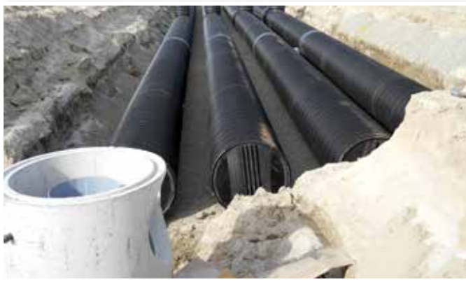
CDS pretreats a rainwater harvesting cistern.
