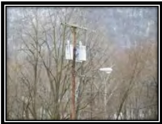
Pole Moutned Transformers
