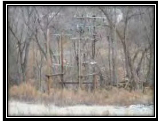
Old Electric Wire Lines
