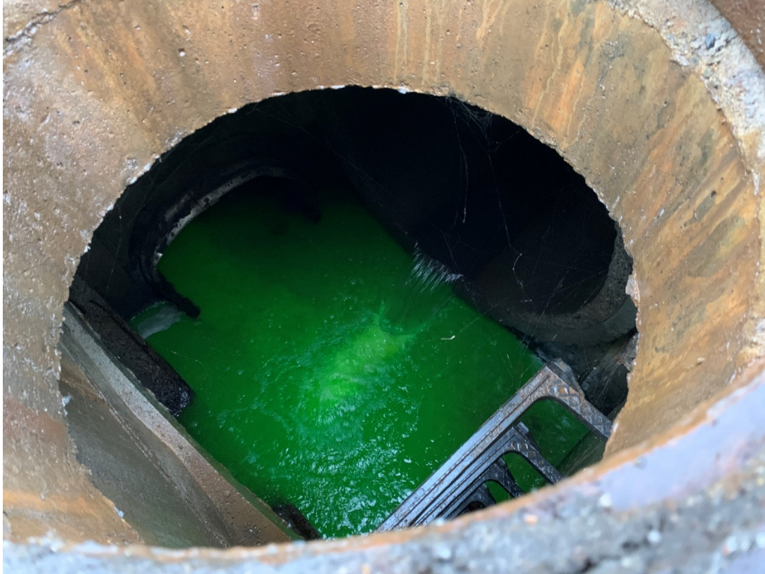
Photo 11: Dye Observed in West Main Street Storm Drain Manhole
