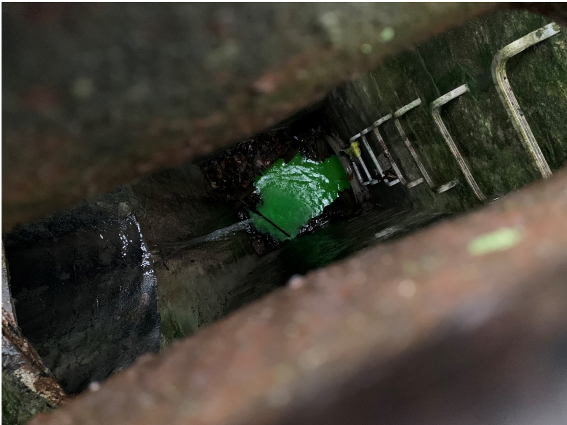
Photo 6: Close-Up of Dye Observed in Bank Street Upgrade Storm Drain Inlet
