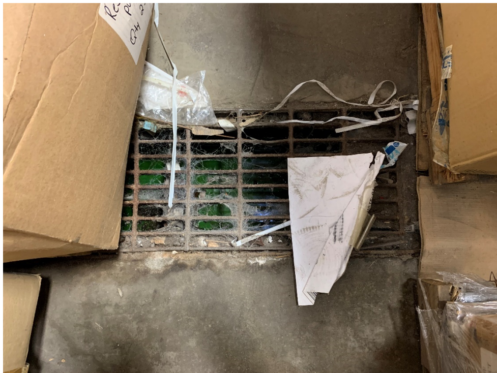
Photo 2: Dye Observed in Floor Drain inside Building
