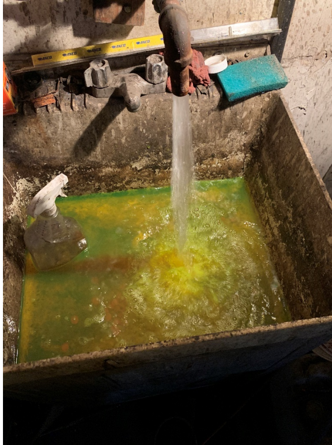
Photo 1: Dye Inserted in Sink
