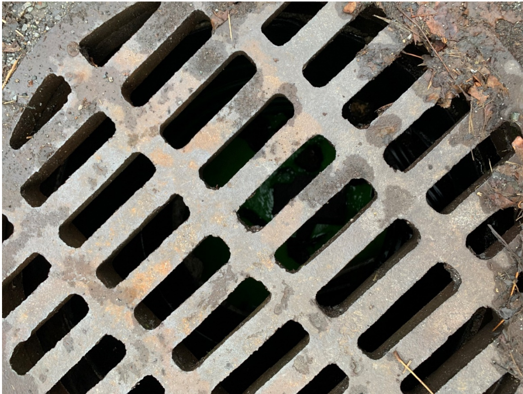
Photo 4: Dye Observed in Rear Storm Drain Inlet
