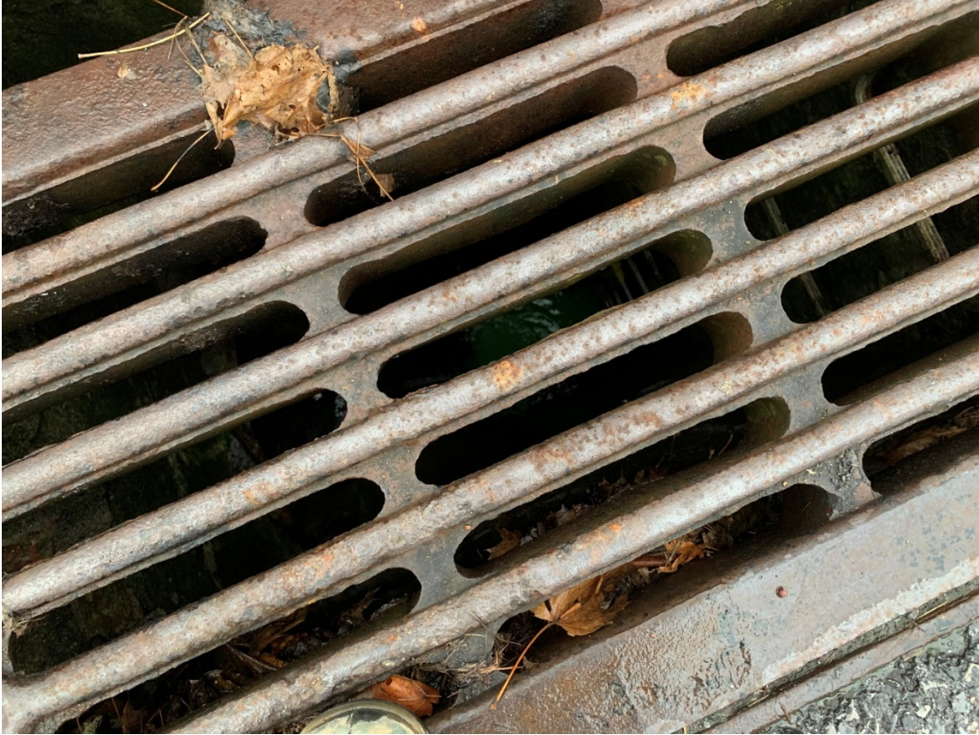
Photo 5: Dye Observed in Bank Street Upgrade Storm Drain Inlet
