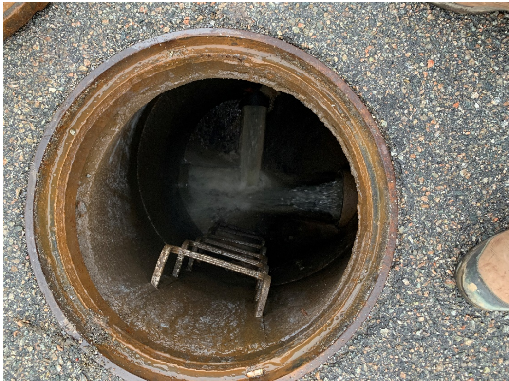
Photo 13: Heavy Stormwater Flow in West Main Street Sanitary Sewer Manhole (Dye Not Observed)
