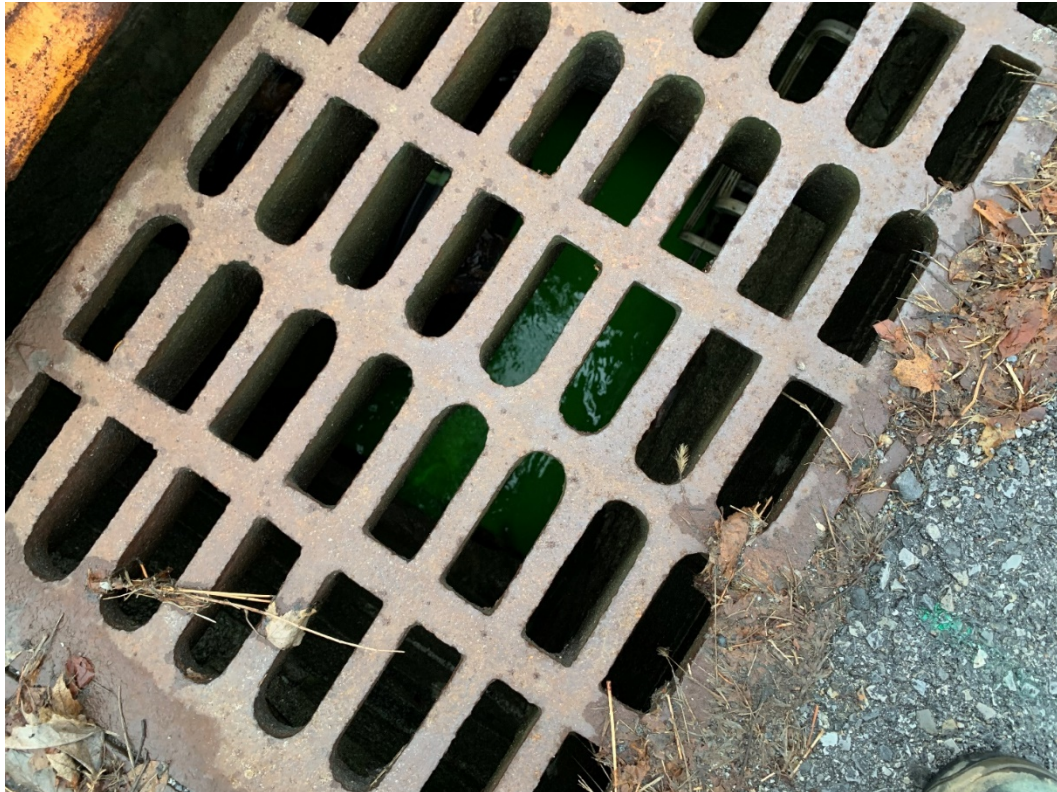
Photo 8: Dye Observed in Bank Street Downgrade Storm Curb Inlet
