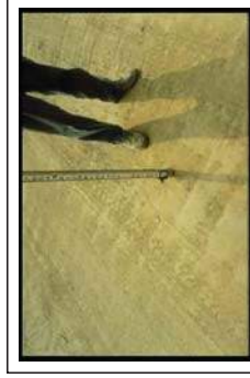
Fig. 3. Construction site with significant compaction of the deep basal till subsoil extends 24 inches below this exposed cut-and-fill work surface.
