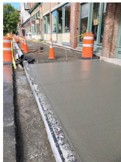
New sidewalks being installed along the east end of Main Street in June 2019.
