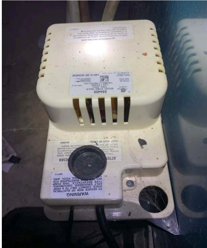
Figure 3: Furnace Condensation Pump in 4 Cross Street
