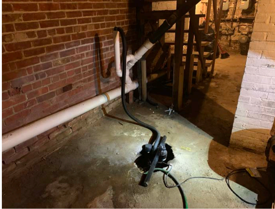
Figure 2: View of Basement Sump Pump and Connection to Sanitary Sewer in 172 Main Street Basement
