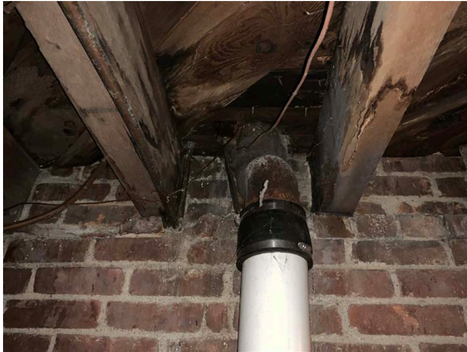
Figure 1: View of Interior Roof Leader in 172 Main Street Basement
