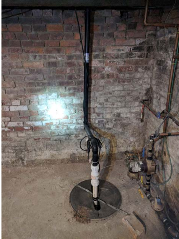
Figure 5 - View of Sump Pump in Basement of Front Building
